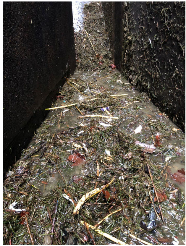
Debris and dead shad on floor at down stream end of dewatering structure.
