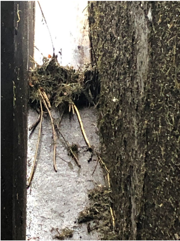
Debris accumulation at top of inclined floor, dewatering structure exit.
